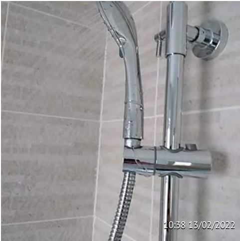
72 Bathroom trade Plumber Leak from handset
