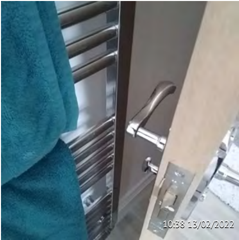
81 Bathroom trade Carpenter Door stop required
